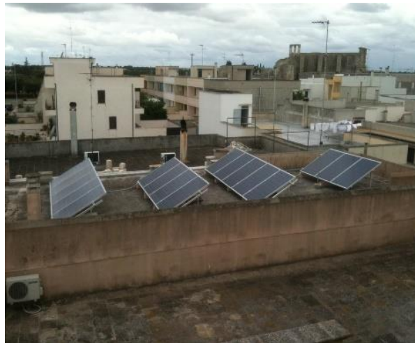
Picture 7: Rooftop photovoltaic energy in Melpignano. Source: Marina Moioli
