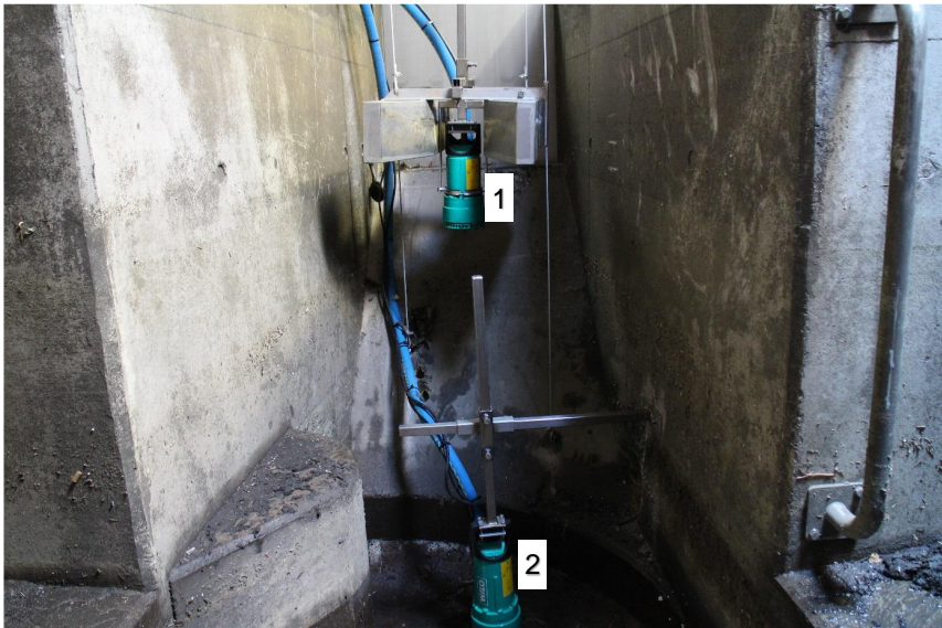
Fig. 4.9: Installed sampling pumps at the stormwater treatment facility RFM Haid, 1 overflow, 2 effluent
